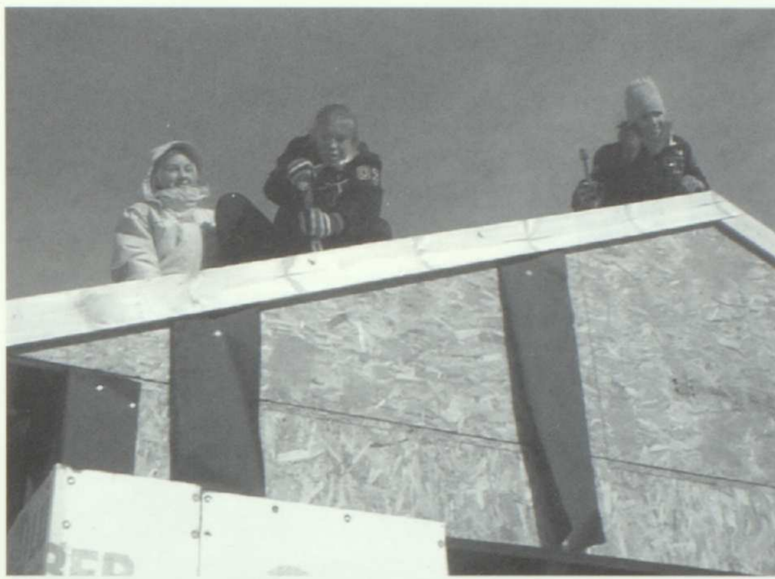
Pounding the finishing nails into the roof are (left to right) Jenny Walker, Anne Young, and Carrie Stanek.
