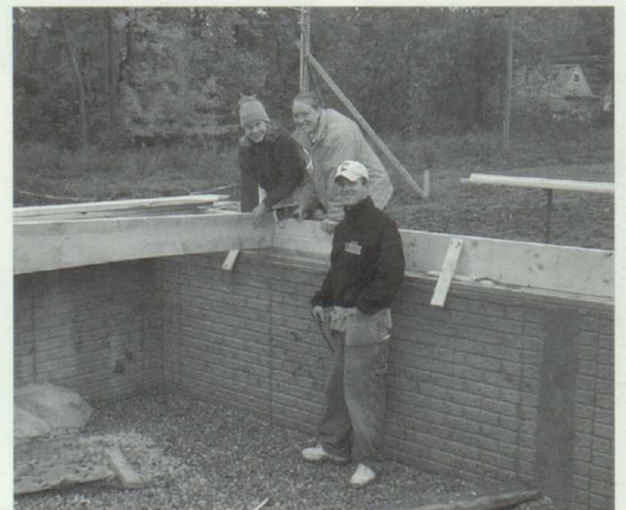
Putting in the floor joists are (left to right) Michelle Massey, Brittany Roeder, and Jason Weale.
